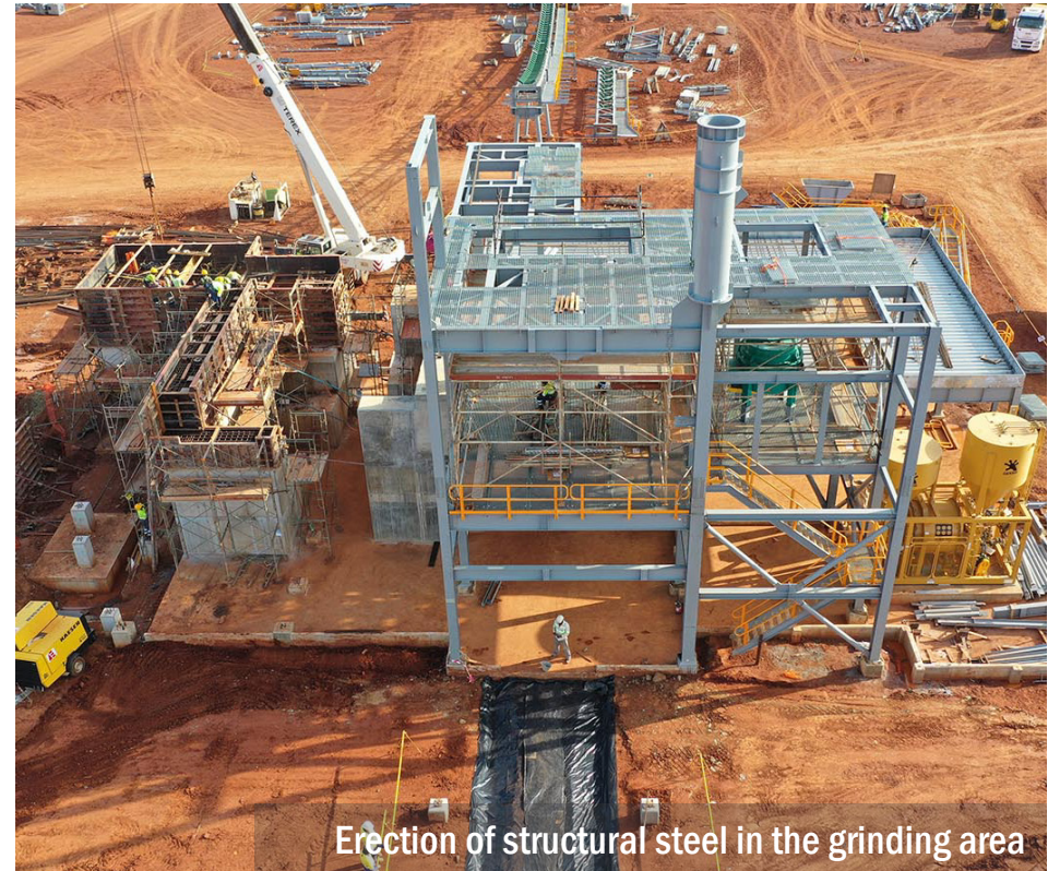
CIL and water tanks erected; thickener assembly and structural steel erection underway
